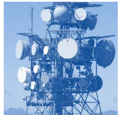
Tower with microwave link antennas (source: arstechnica.com)
